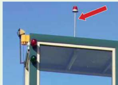
Emergency siren and lighting devices provided at the supervisor box.
